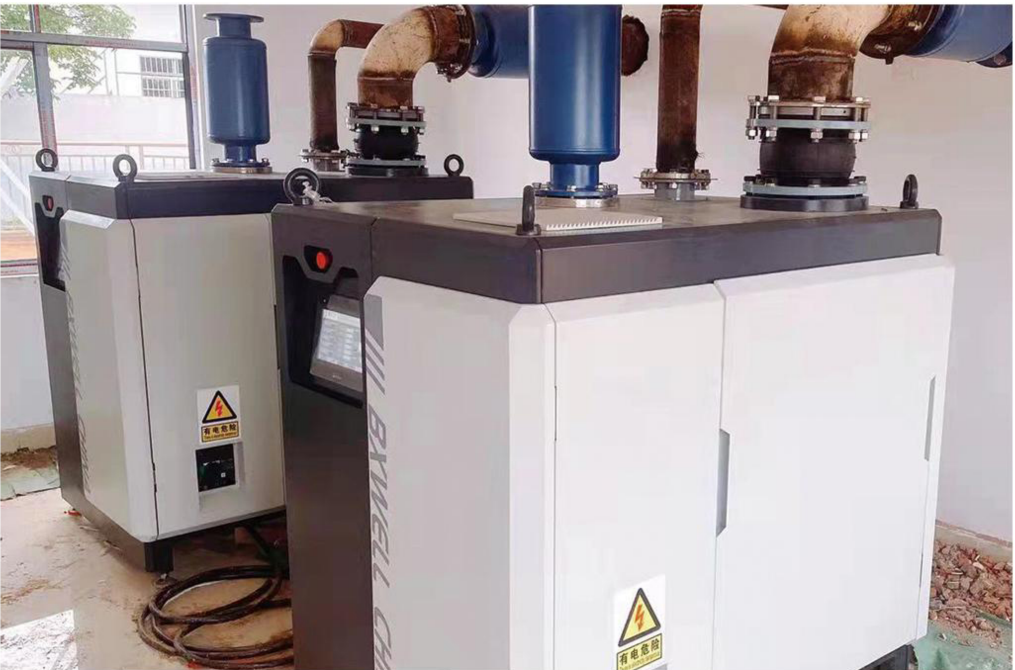
A sewage plant in Qinzhou City, Guangxi
