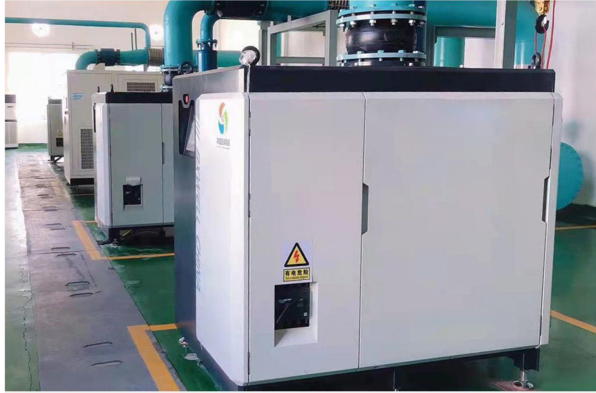
A new materials company in Inner Mongolia
