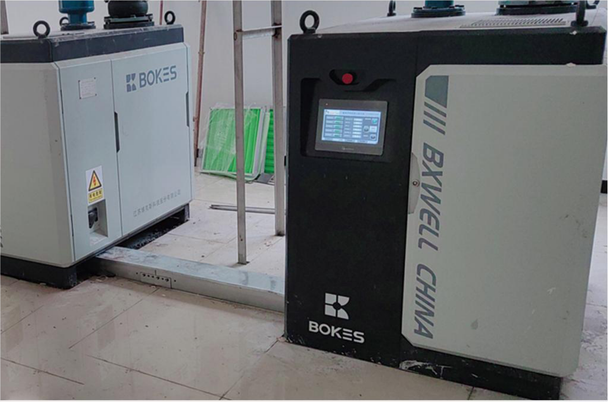
A sewage treatment plant in Hubei
